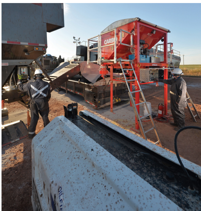
Figure 2. The CARBO production services team ensures that each production assurance treatment is executed as designed.
