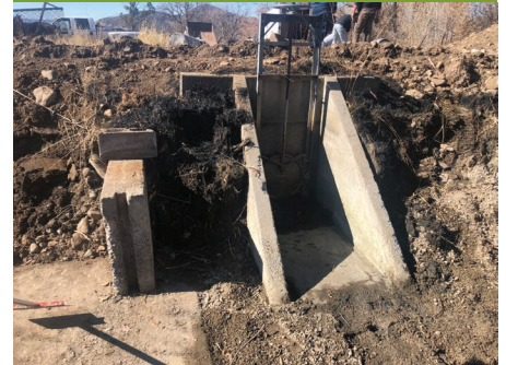
Poor soil conditions allowed erosion and build-up of debris at the canal gate and check gate.
