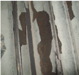
Fin cleanliness, pre-blast
